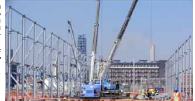
Civil engineering operations have already begun and the first engines will arrive on site next May. Handover of the completed plant is scheduled to take place in December 2012.
