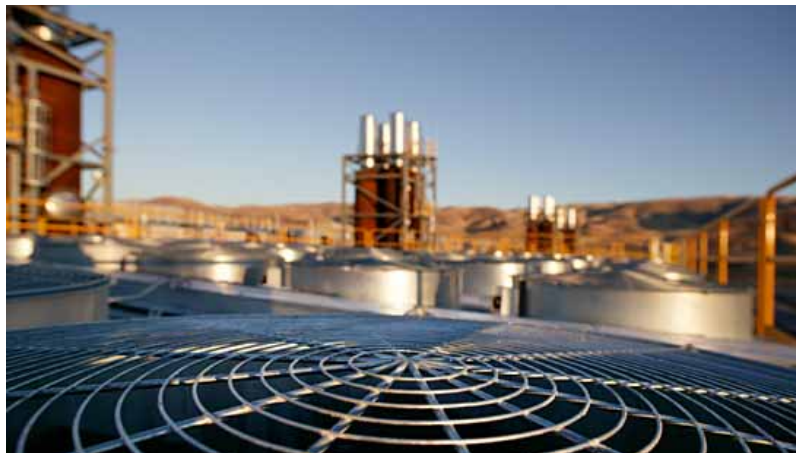
The Quisqueya I combined cycle plant will be located in San Pedro de Macoris, Dominican Republic.
